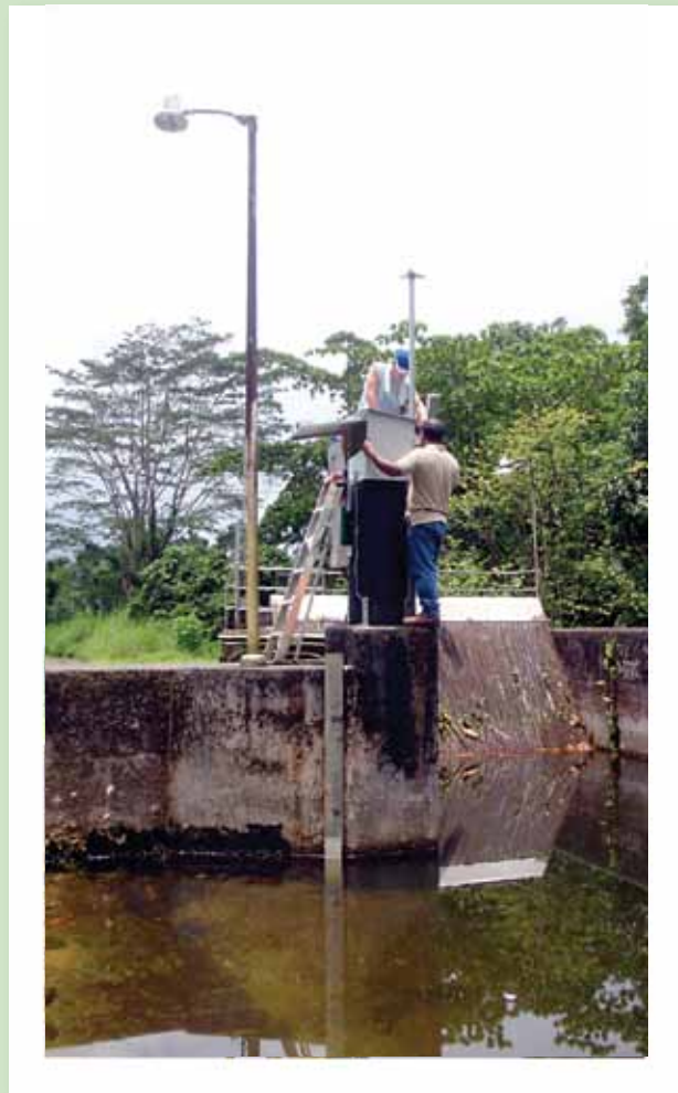
Nanipil Weir and hydro electric intake finalising water level recorder, gauge board and raingauge
