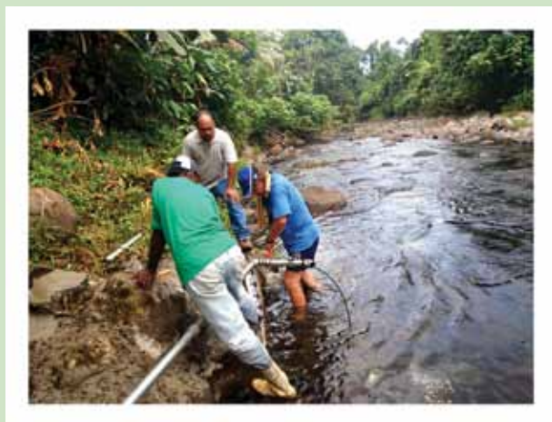
Construction activities installing sensor line, Senipehn River December 2009 looking downstream. This river is equally responsive to heavy rain as the Nanipil. Note the well armoured bed, dense indurated volcanic boulders typical of Pompei Rivers with little fine material.
