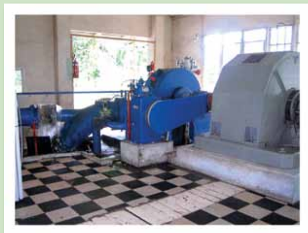
Samoa Electricity Authority Vaisigano Hydro Power Plant
