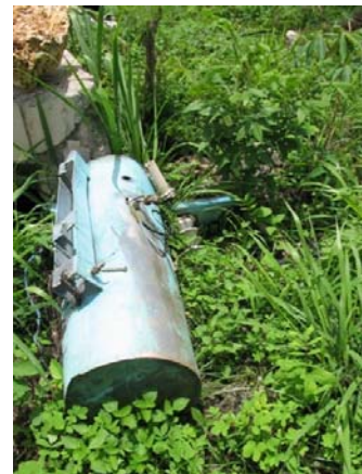
Broken down transformer
