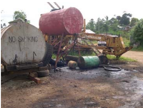
Leaking oil and gasoline seeps into the ground leaking oil containing PCB
