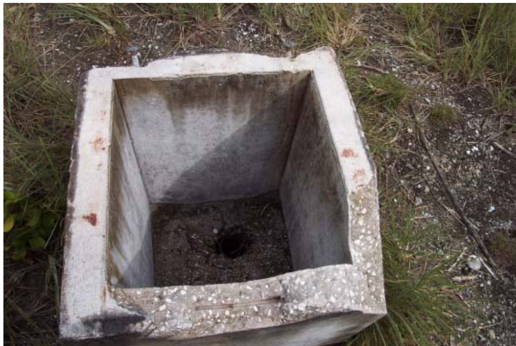
Figure 21. Vandalism to infrastructure is a reoccurring problem in water reserves. This was Bonriki salinity monitoring borehole BN4B. The steel lid has been smashed off and the piezometer tube and salinity monitoring tubes have all been removed.
