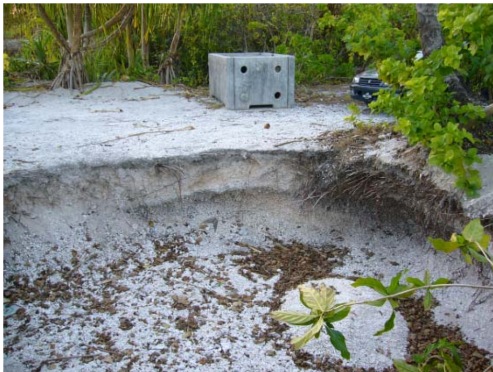
Figure 14. Sand and gravel mining has completely destroyed salinity monitoring borehole BN 16 (beside PS 7), one of the oldest and the deepest borehole in Bonriki.
