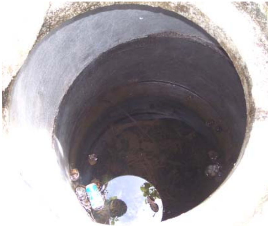
Figure 20. Rubbish thrown down the terminal well of PS 7.
